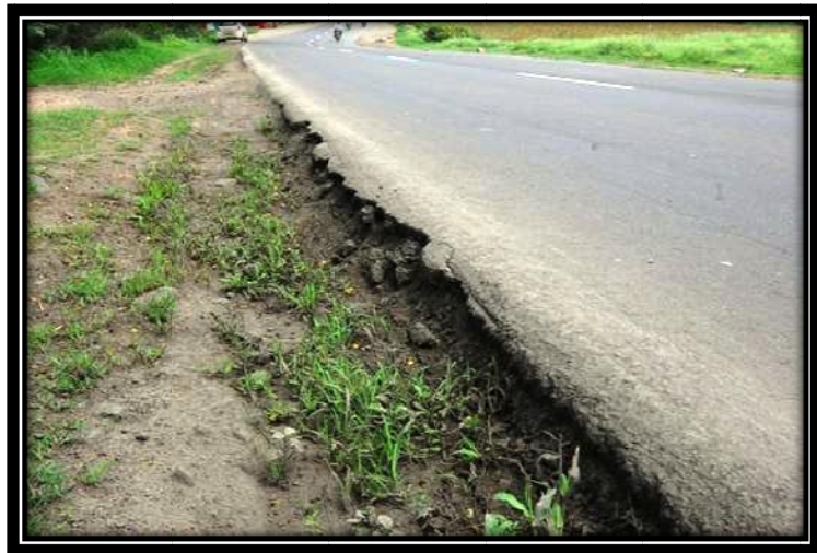
A step of almost a foot between the pavement and the shoulder, on NH-50.
