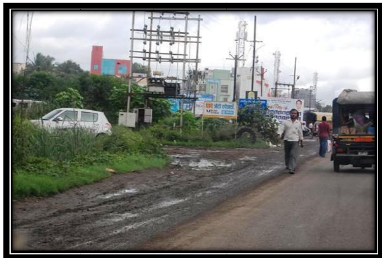
A lane joining NH-50 at right angle. Also notice the state of the shoulder, forcing pedestrians to walk right on the National Highway!
